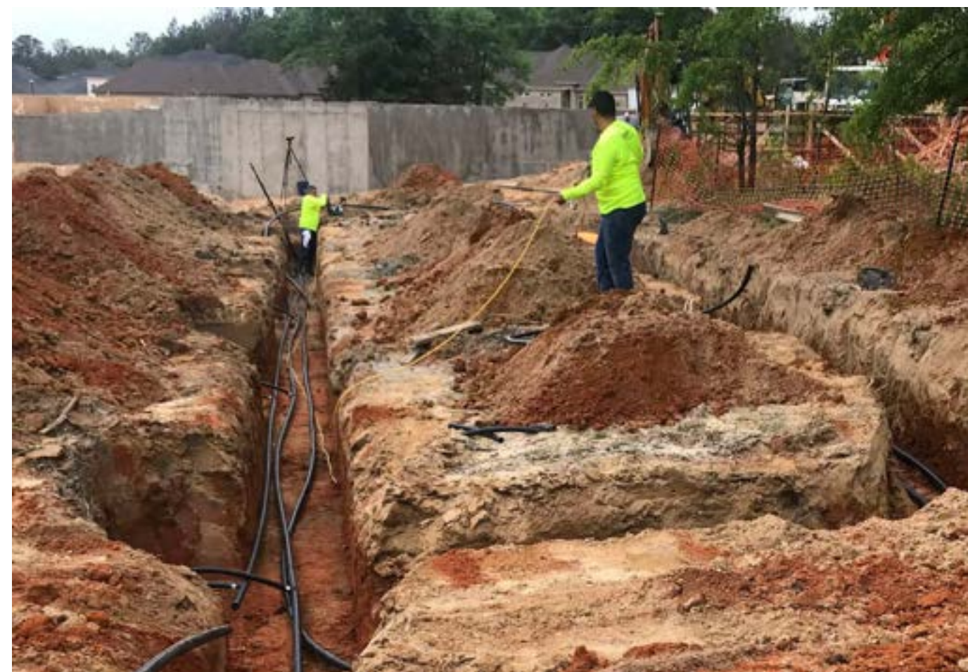
Connections in the 7-well field are made along a U-shaped trench, so that all of the plastic piping will be 4 feet below the finished ground surface. Two plastic pipes will connect the well circuit with the house just beyond the camera tripod, at the far end of the trench in front of the concrete foundation.
