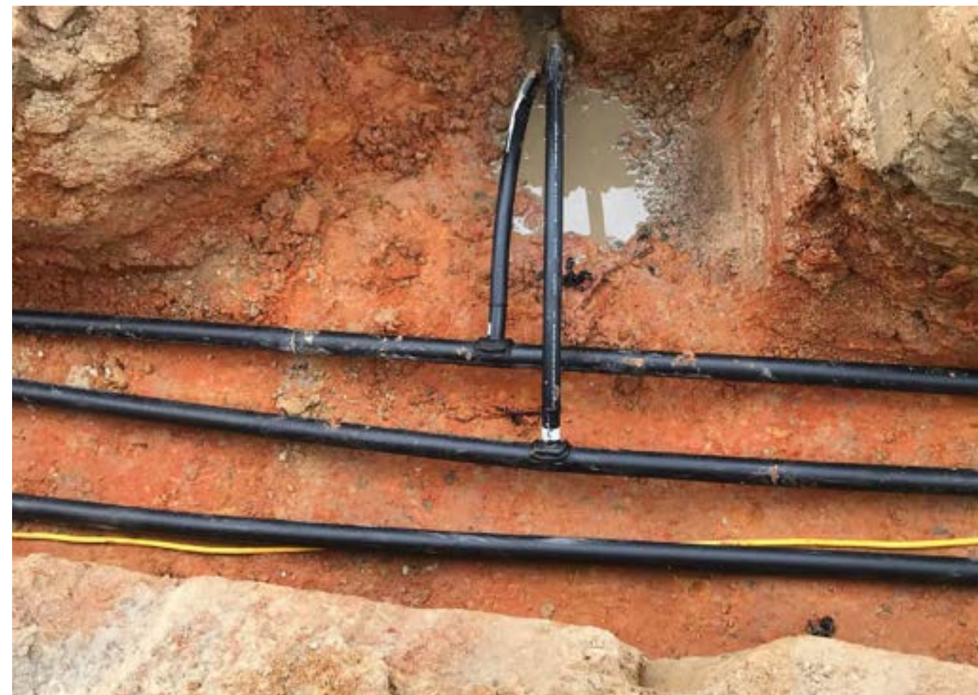
The ends of a well loop are thermally welded to the connecting pipes to form a circuit with the other 6 well loops and with the geothermal system in the house.
