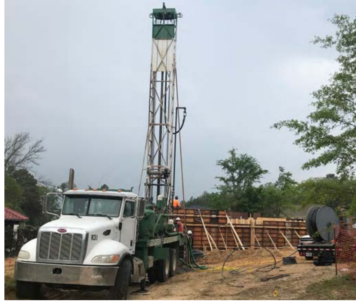
The geothermal wells were drilled using the same sort of rig used for water wells. Forms for the concrete foundation of the house are in the background.
