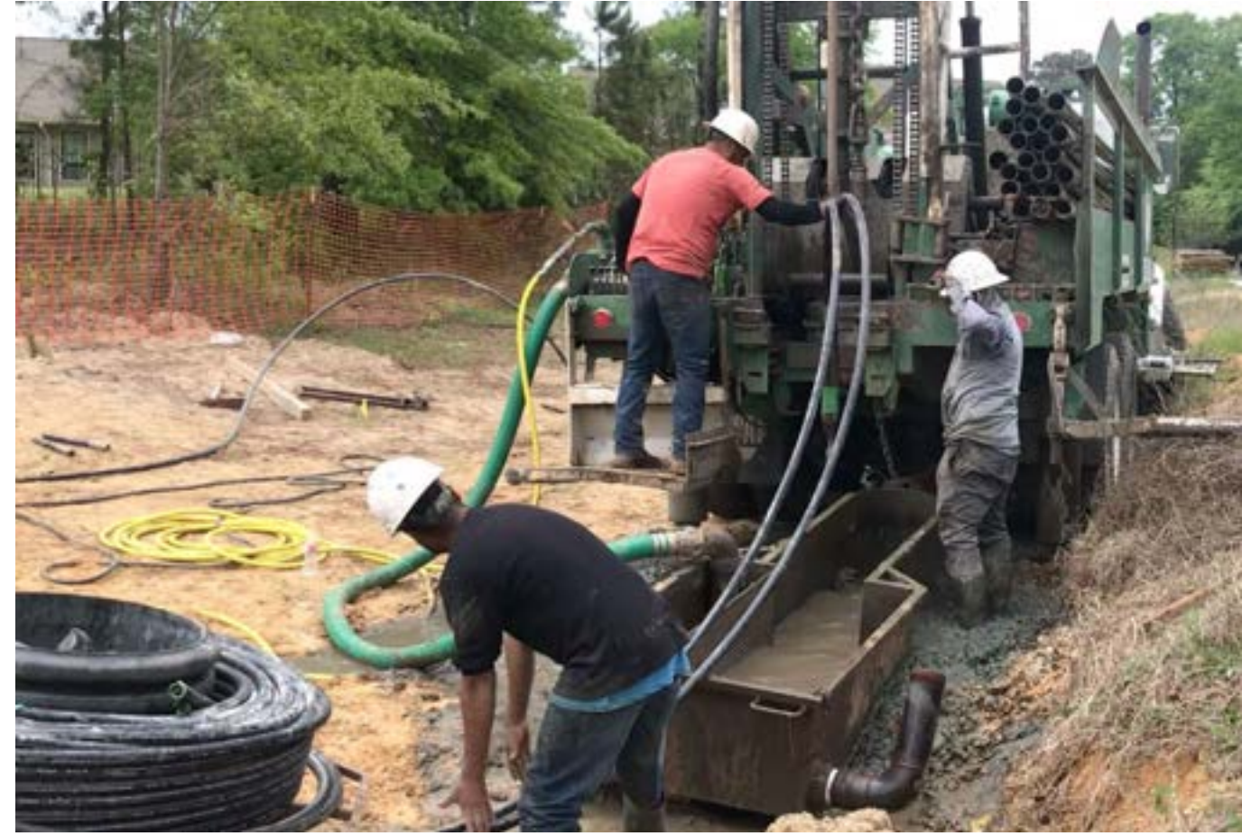
A loop of 1" HDPE tubing filled with water is lowered into one of the geothermal wells using the rig cable.
