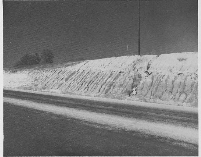
Fig. 31. Locality 48. A trough-shaped clay-filled channel is present in the Eagle Mountain Member of the Paluxy Formation. The channel appears trough shaped in cross section and exhibits distinct upper and lower contacts with the adjacent sands. Note the distinct color, bedding, and lithologic changes in the far left side of the photo. The clay that fills the channel is gray and contains large amounts of sand and carbonized plant remains. The adjacent sands are white, fine to medium grained, subrounded to subangular, and poorly to well sorted.
