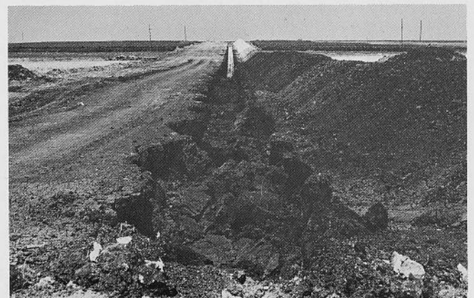
Fig. 19. Low slope stability in vertical walled excavations is indicated in this photograph of the Houston Black clay. Major slumping did not occur until after a rain. The whiter area toward the top of the photograph is an Austin soil and demonstrates the rapid soil changes possible within similar rock types.
