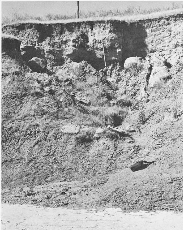
Fig. 2. Austin Chalk-Taylor Marl contact (Loc. 2, Plate I). Three distinct rock types are present: the white area at the bottom is the Austin Chalk (high bearing capacity), the gray area extending vertically to the top of the shovel is the Taylor Marl (low bearing capacity), and the gray and black stratified area above the shovel is alluvium (low to moderate bearing capacity). Note low slope stability of the Taylor compared to the partially cemented alluvial gravels.
