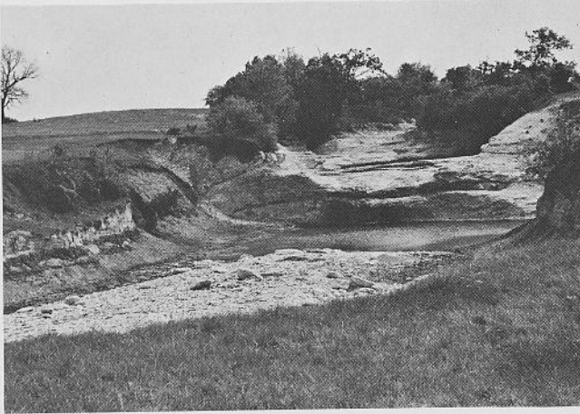
Fig. 10. "Upper" Austin Chalk in fault contact with Taylor Marl in the spillway of Lake Waxahachie (Loc. 1). Changes in soils, slope stability, bearing capacities, and other engineering properties can occur quite abruptly as a result of faulting. Note Taylor Marl slumping immediately adjacent to the fault contact.
