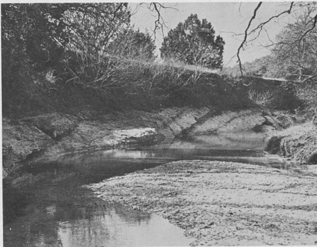
Fig. 4. Lower Austin on White Rock Creek, Locality 2. This location is about 100 yards north of Gholson Road. Notice the extreme dip in the Austin Chalk causing alternate beds of marl and chalk to lie just under the alluvium. Support strength in locations such as this will be controlled by the weaker marl beds. Areas like this require extensive site listing to determine the extent of these near vertical alternate beds and the extent of faulting and jointing.
